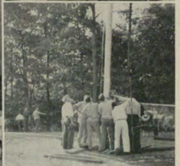
Deltasig Lodge in mid-winter . . . Stag week-end . . . Snake Rives . . . Valentine Dance . . . putting up the flagpole in front of the lodge.
