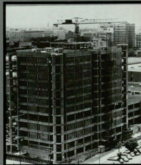
Middle: As new buildings were completed, construction on the plaza system began, which would link together the university through an elevated walkway.
