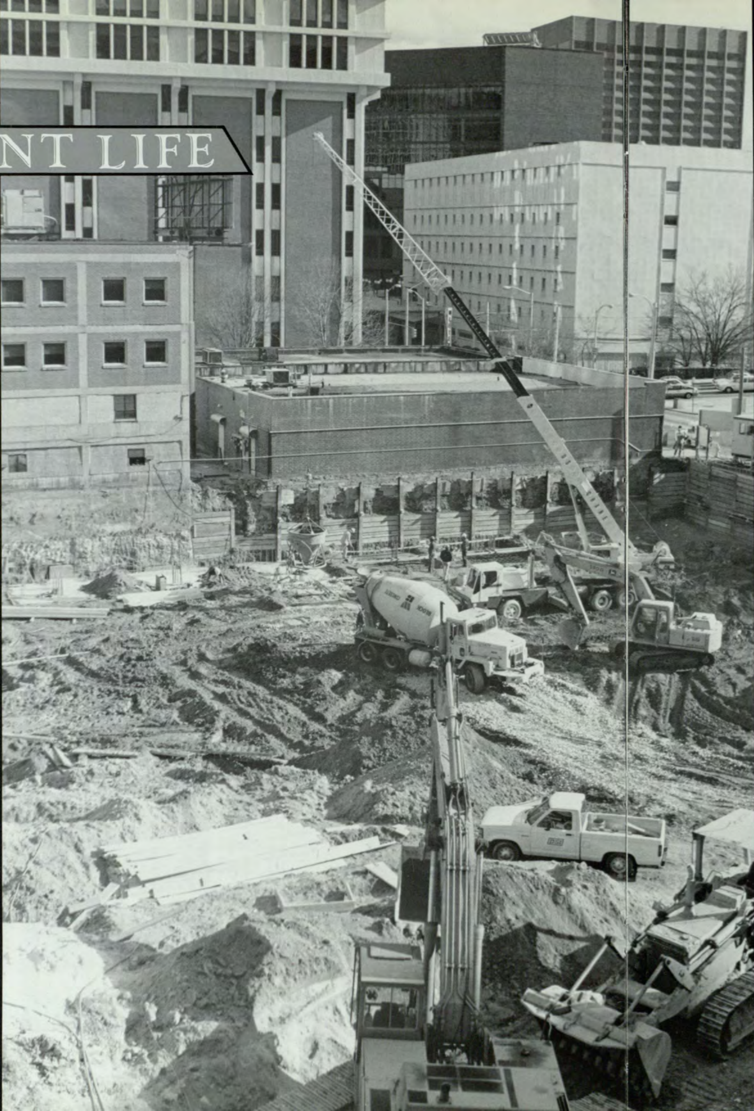
BEGINNING A STRONG FOUNDATION — Construction of the new Science Building on Decatur Street began in January. Photo by David Newton.
