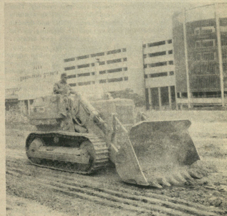
A bulldozer began clearing ground last Monday beside the BA Building for new pavement on the G lot. Among the features of the area destined for destruction are some street cobblestones from Atlanta's early days and a grove of old cottonwood trees beside the business school.
